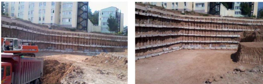
Fig. 2. A view of the retaining system at the last stage of the excavation
