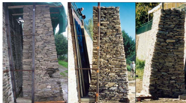
Fig. 2. Experimental wall of Villemus et al. (2007) (a) Before loading, (b&c) After loading
